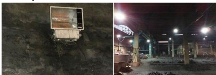
(L) Existing lighting; (R) energy efficient lighting
