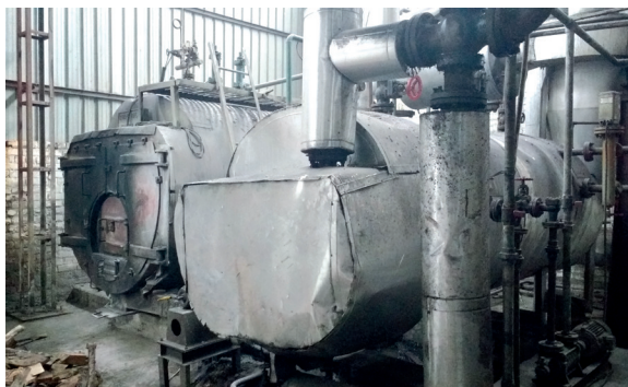
Solid fuel fired boiler and thermic fluid based steam generator
