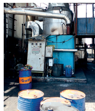
Thermic fluid heater
