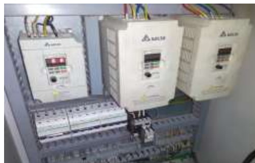
VFD for cranes and hoist motors
