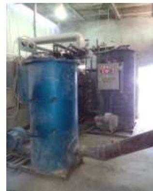
Gas fired thermic fluid heaters
