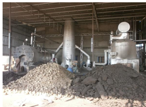
Boiler and thermopac
