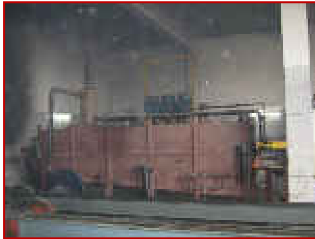
Figure 3.8: Operation of Energy efficient reheating furnace
