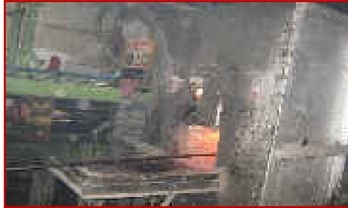
Figure 3.7: Operation of conventional oil fired Billet heater
