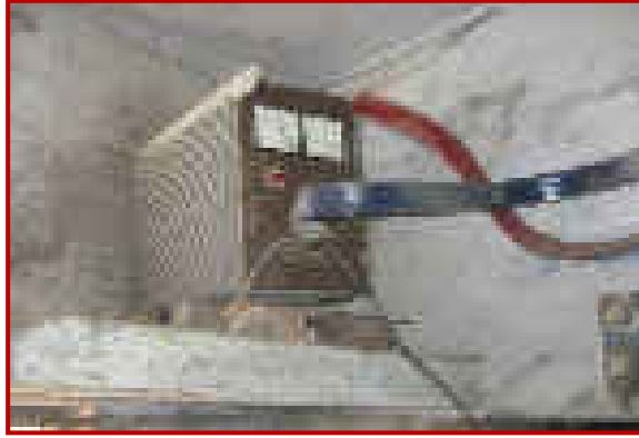
Figure 3.12: Operation of energy efficient rectifier in electroplating unit
