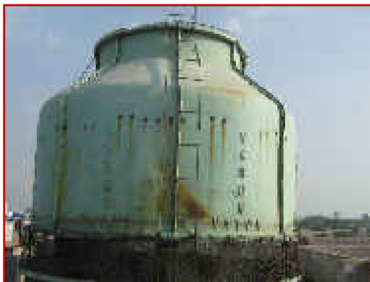
Figure 3.13: Operation of cooling tower in typical Brass extrusion unitError! Bookmark not defined.
