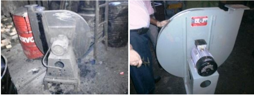
Combustion air blower: L- Low capacity; R- Optimum capacity
