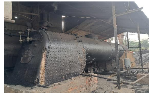
Old inefficient boiler
