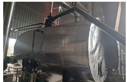
Energy efficient boiler
