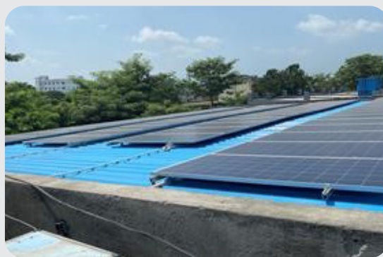
Figure 1: Solar rooftop module
