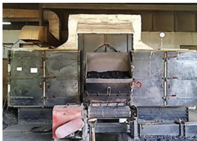
Figure 5. Coal-based hot air generator (HAG) for drying
