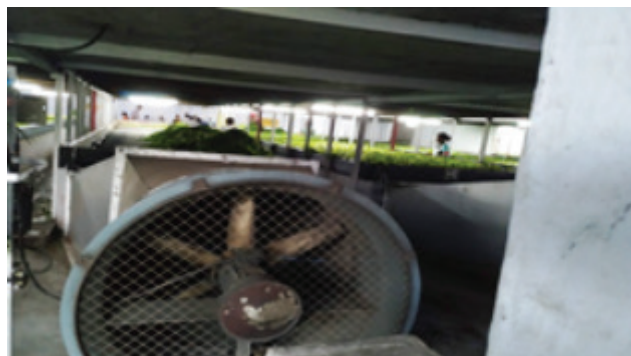
Figure 2. Axial fan attached to withering bed
