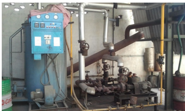
Thermic fluid heater
