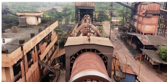
Rotary kiln in DRI plant
