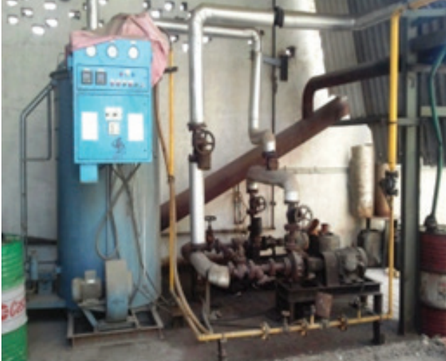
Thermic fluid heater in chemical industry – mapped under BEE program
