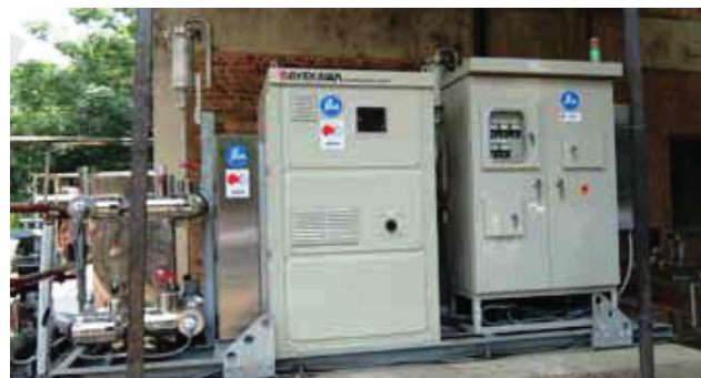
EHP system implemented in a dairy plant, Chandigarh
