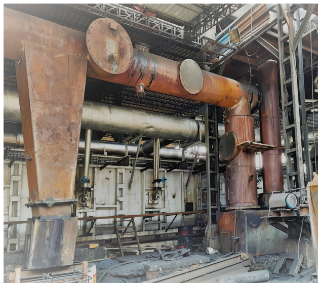
Coal gasifier system in steel rerolling mill
