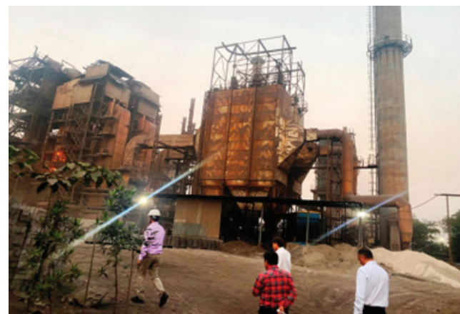
Waste heat recovery boiler (WHRB)
