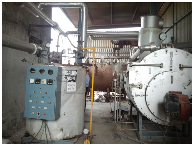
Thermic fluid heater
