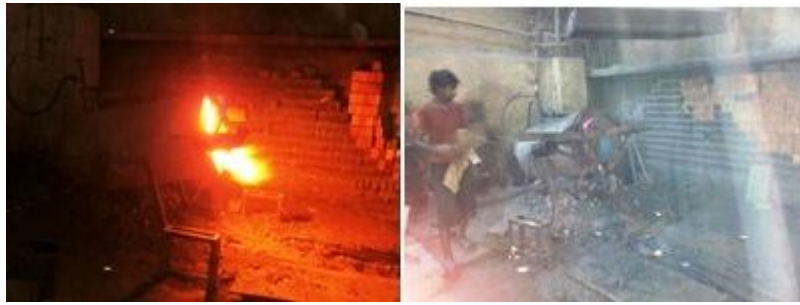
(L) Damaged lining in existing FO-fired furnace; (R) furnace after relining
