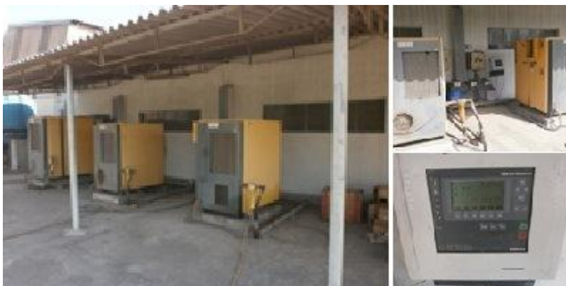
(L) air compressor system; (R) with sequence controller
