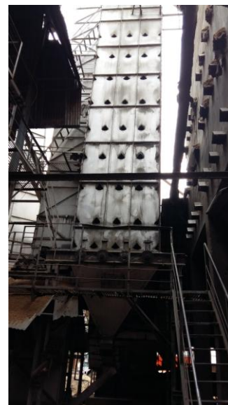
Counter flow hot air dryer
