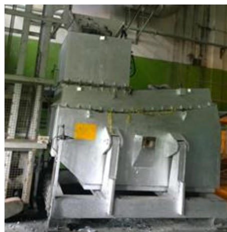
Reverberatory/ Slakner furnace
