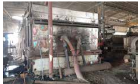
Furnace control system
