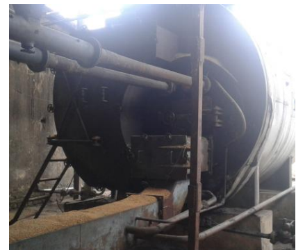
Rice husk fired boiler
