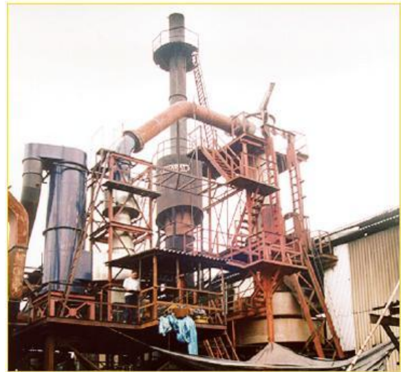
Demonstration unit at Howrah
