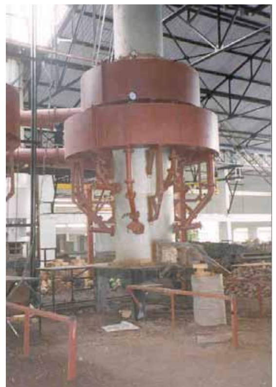
Divided blast cupola installed at a foundry in Rajkot
