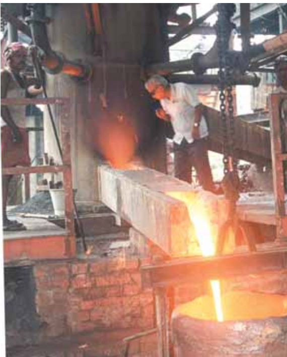
► Commissioning of the demonstration plant at Howrah
