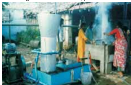
Biomass gasifier for thermal applications
